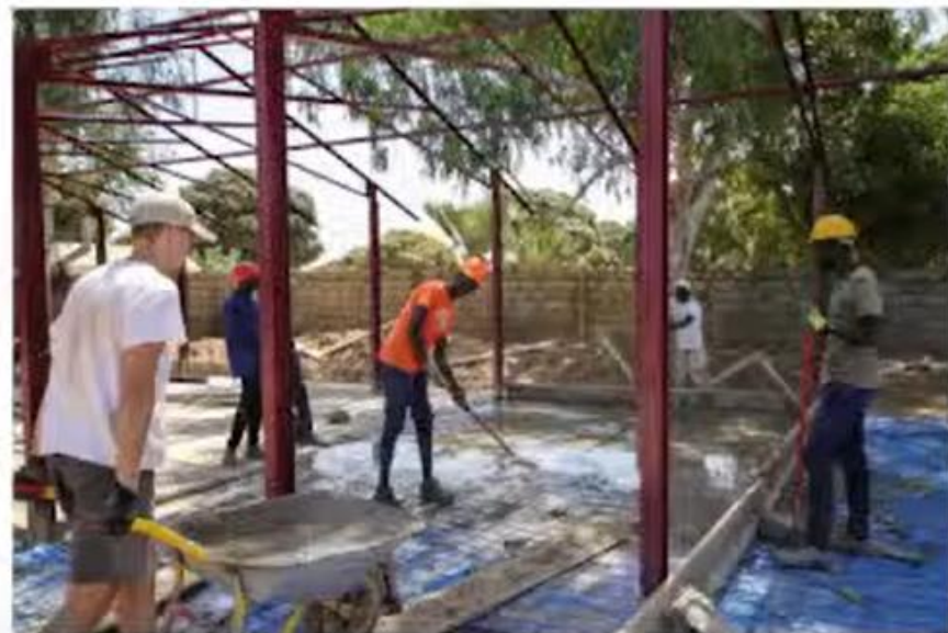
// Robno mešanje betona in betoniranje talne plošče // Hand mixing of concrete and casting the floor slab
