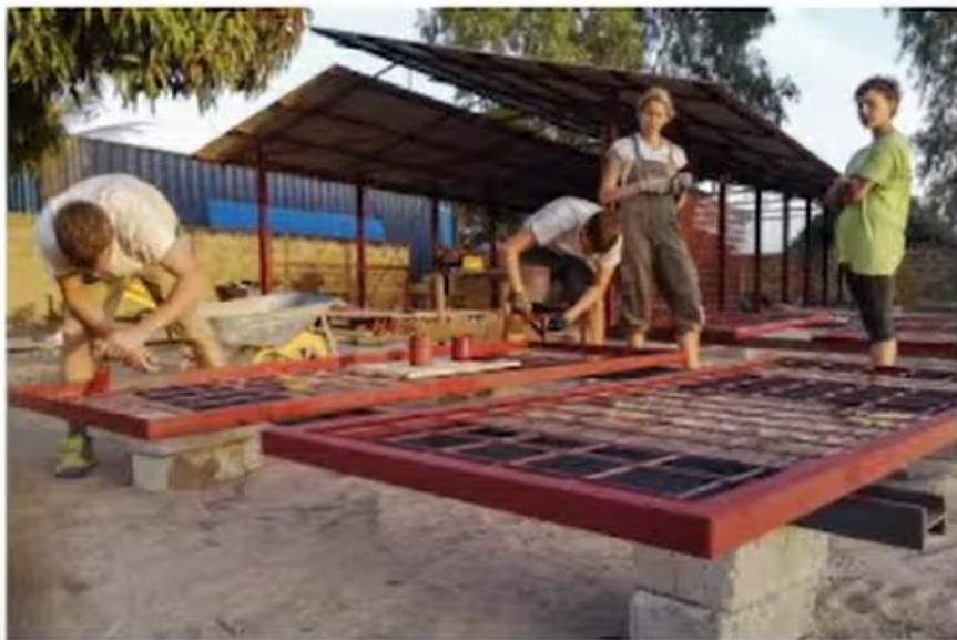
// izdelava drsnih panelov - varjeni okvirji iz "L" profilov in armature mreže // Manufacturing of sliding panels - welded frames from "L" profiles and reinforcing mesh
