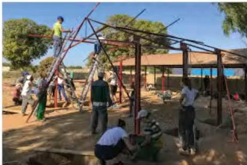
// Dvigovanje jeklenih okvirov in umeščanje stebrov v točkovne temelje // Erecting of steel frames and fixing of pillars into foundations
