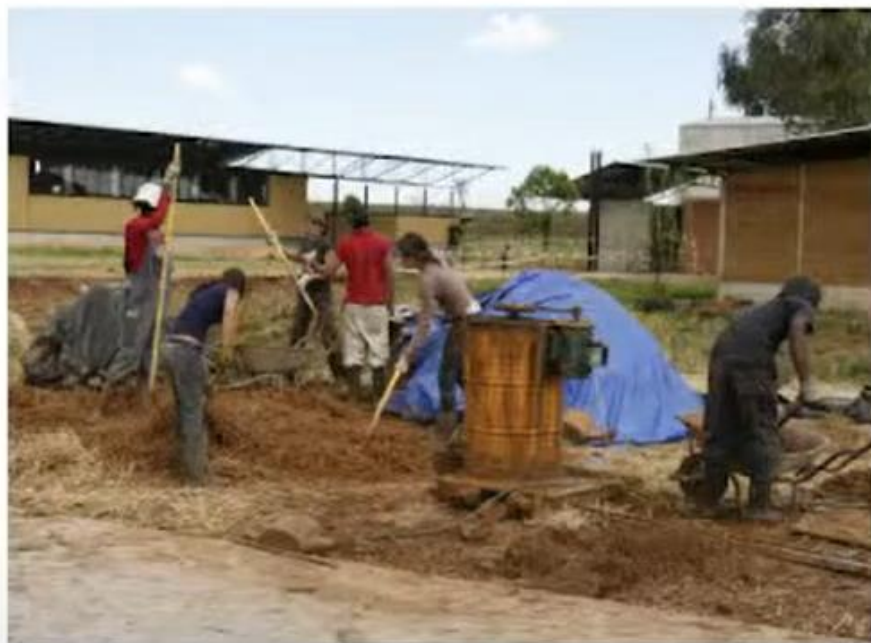
// Priprava mešanice slame in gline za butanje sten // Making of straw and clay mixture for ramming the walls
