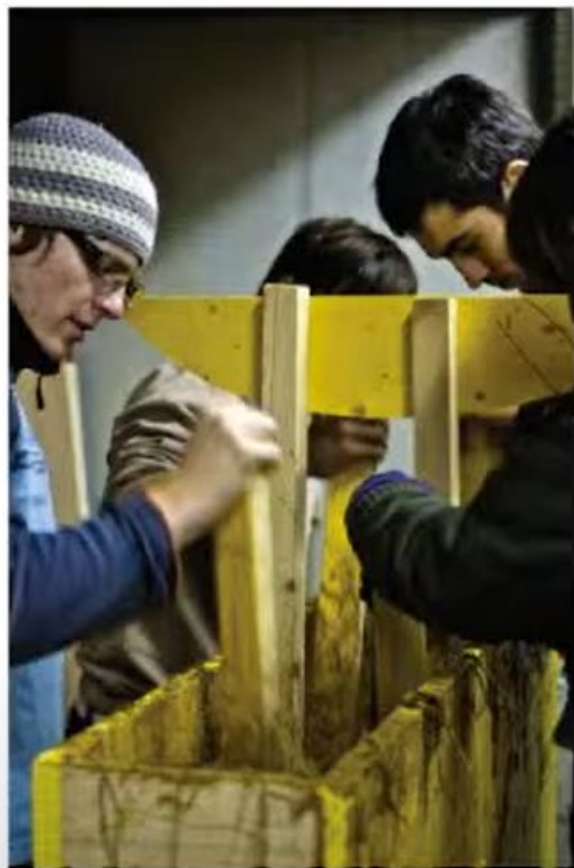
// Učenje butarja slame in glino, klet Fakultete za arhitekturo, 2009 // Learning of ramming straw and clay, Faculty of Architecture, 2009
