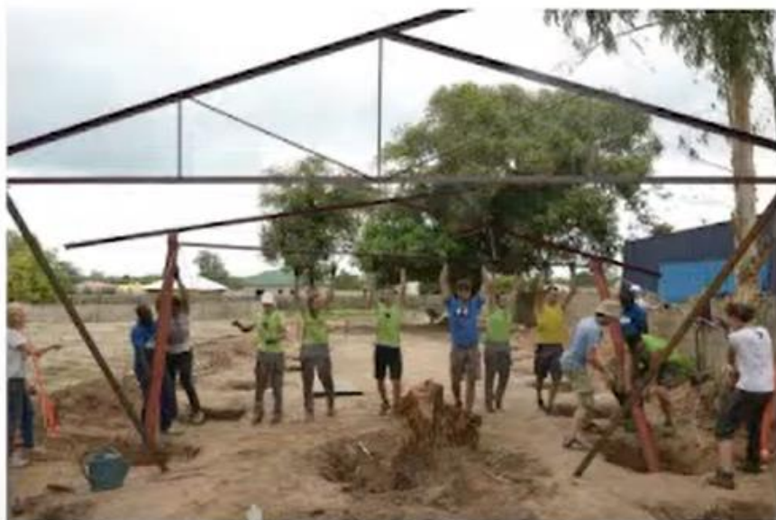
// Dvigovanje jeklenih okvirov in umeščanje stebrov v točkovne temelje // Erecting of steel frames and fixing of pillars into foundations
