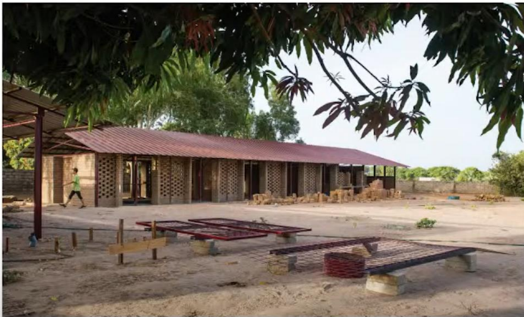
// Izdelava drsnih panelov - vrat učilnic Male šole // Manufacturing of sliding panels - doors of classrooms of the Nursery School
