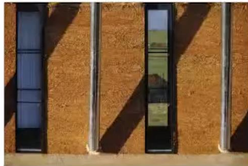
// Južna fasada - okna in masivna stena z zračniki za iztek mraznega zraka // Southern facade - windows and massive walls with vents for suction of cold air
