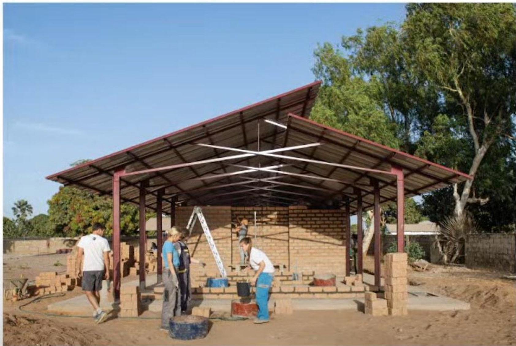
Il Zidanje cik-cak sten z namenom izboljšanja njihove stabilnosti Il Zig-zag bricklaying of the walls with the purpose of their stabilization
