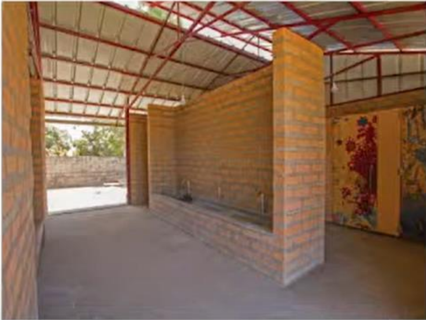
// Sanitarje - veliki urivodnik in kabine, poslikane s poslikavami otrok iz sosesčine // Lavatories - large wash basin and toilets with doors, painted by neighborhood kids
