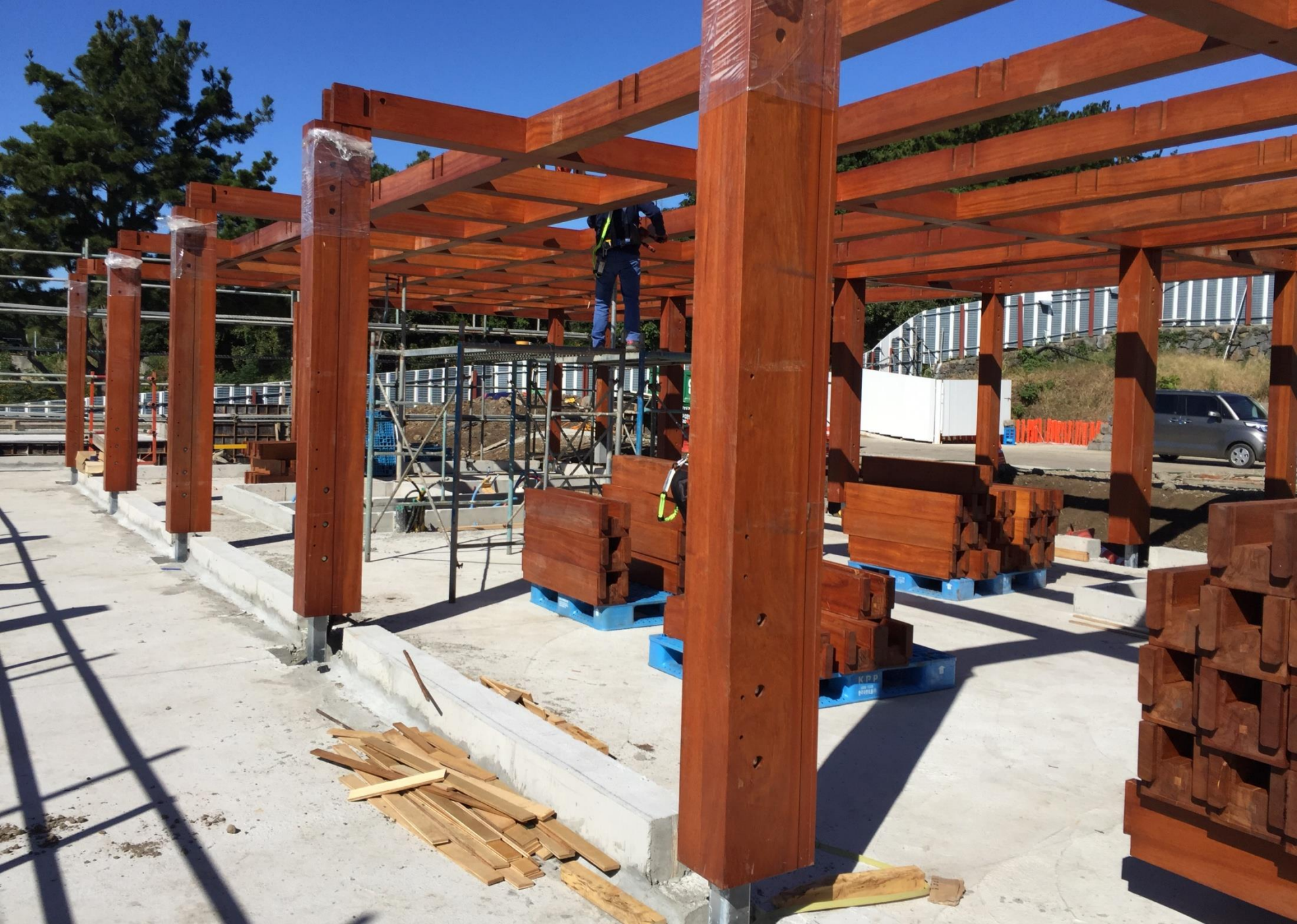
TOC TOC | TIMBER ARCHITECTURE IN FOCUS AS & CC | Jeju Tea House | 2014 - 2018 | Jeju Island, South Korea
