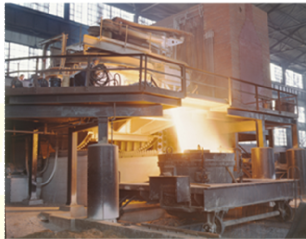
Electric Arc Furnace
