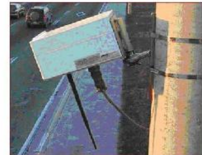
RTMS (Remote Traffic Microwave Sensor) radar Camera Sensors
